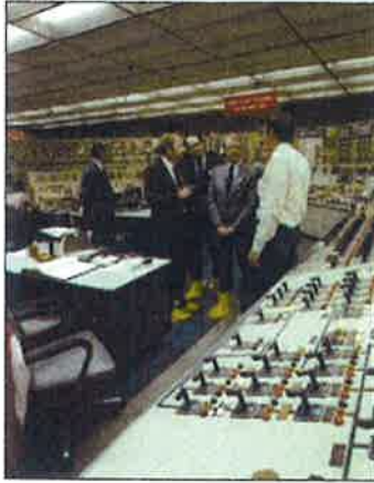
President Jimmy Carter briefed by James R. Floyd, supervisor of TMI-2 operations, with Harold R. Denton, director of the Office of Nuclear Reactor Regulation in the Nuclear Regulatory Commission. This control room design was complete in the late 1960s, before construction began in 1970.
