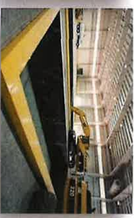
Solids / Wastewater Treatment
