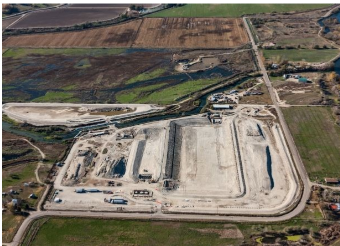
Work on the Dixie Drain phosphorus removal facility on the Lower Boise River. Photo from the Department of Environmental Quality.
