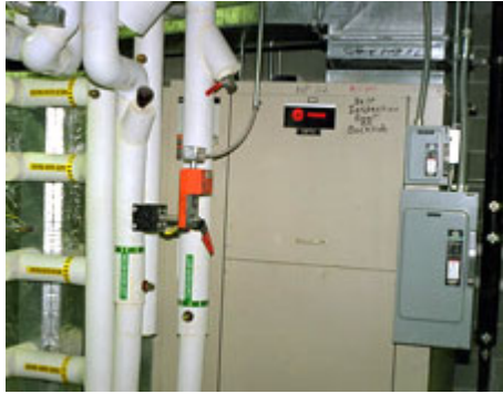
Ground-source heat pump (Source: NREL)
