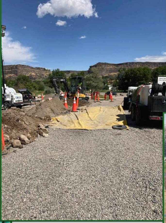
Water and Electrical Utilities
