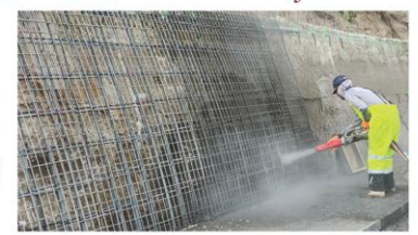
Construction specialist applies shotcrete, a mix of cement, sand, and aggregate mix pneumatically projected through a hose at high velocity onto the walls of the North Side main canal below Milner Dam. (Photo courtesy North Side Canal Co.)
